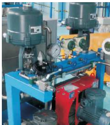
On site application of hydrogenation flowmeter
