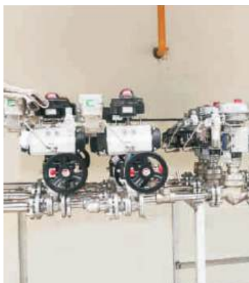
On site application of hydrogenation flowmeter
